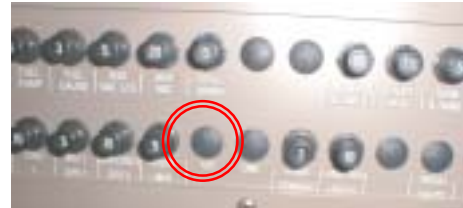
Figure 2-4 Circuit breaker location (Typical)
